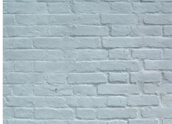
Painted brick should be kept painted. Removal could cause permanent damage to the underlying masonry.
