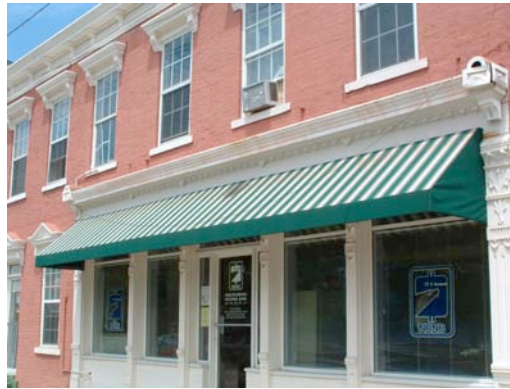
Closed-end awnings are also appropriate. Awnings should be well above head height and should cover only the transom. Leave cornices and decorative details exposed.
